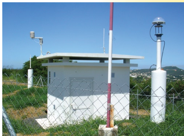
Located in Normandie (Nouméa), this antenna (co-located with a DORIS station) is part of the future network that will include 15 RTK GPS reference stations throughout the main island.
