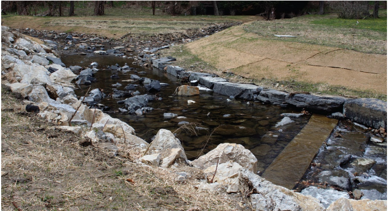
A residential work in progress: an attempt to re-create Mill Creek's desire for a gentler bank along its steeper side, with regrading and seeding in the floodplain. Some hardscaping remains, but damage will be less severe with reduced restriction of the creek's flow.
