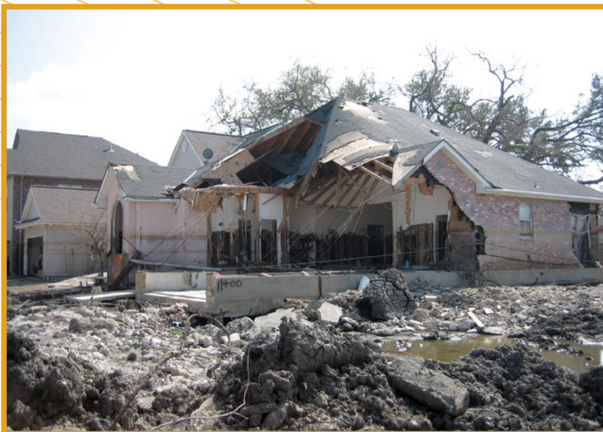
One of the many homes damaged by flowing water at the 17th Street Canal breach.
